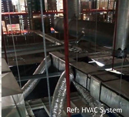
Ref: Cleanroom Vents
